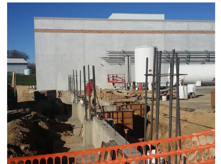
Slow but sure, the project is progressing. We're building a strong foundation in preparation for a great future.
